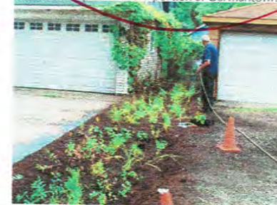
▲ Above photos show commercial and private residential bioswale and rain garden interventions
