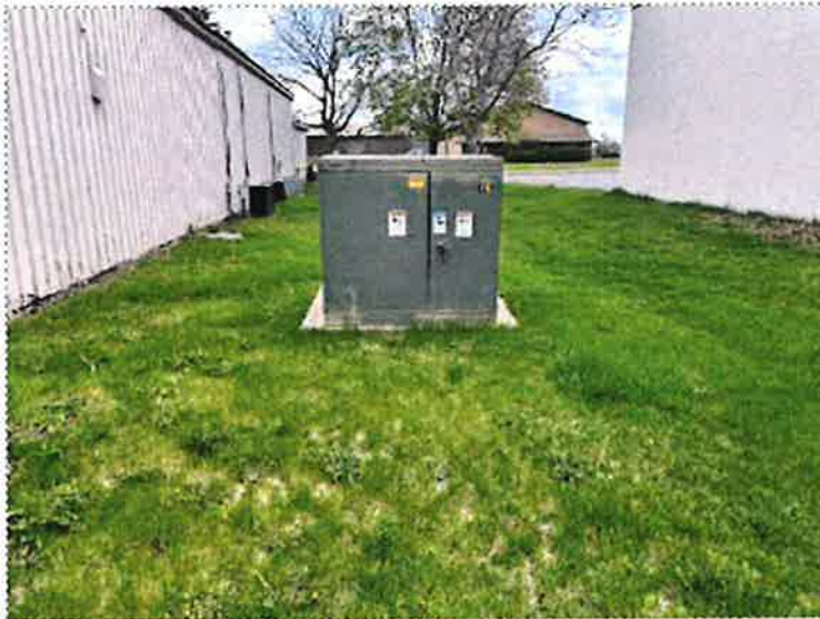
12. View of pad-mounted transformer along western subject property boundary
