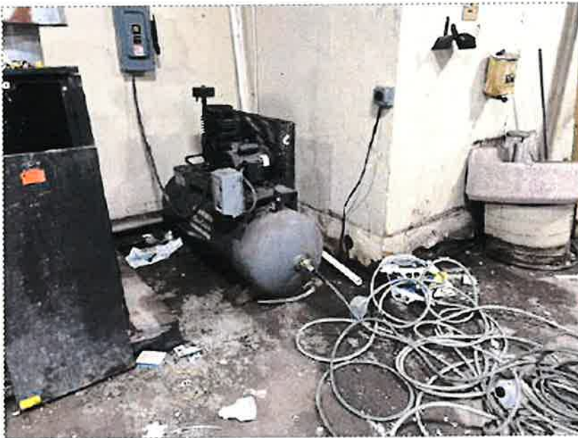
26. View of air compressor and minor concrete staining
