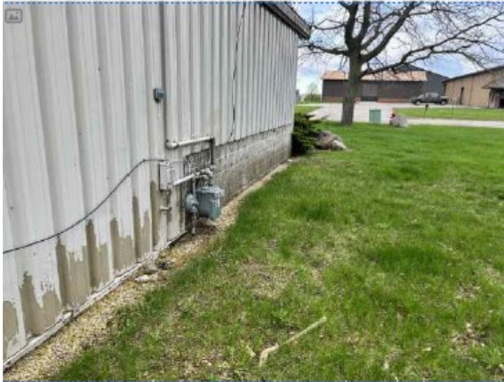
13. View of natural gas connection at southeast building corner
