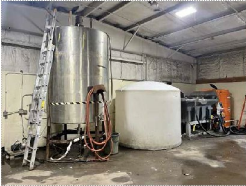
27. View of freshwater stainless steel tank and saltwater poly-tank
