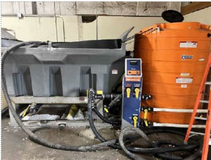
28. View of brine solution machine - grey salt hopper and orange brine water
