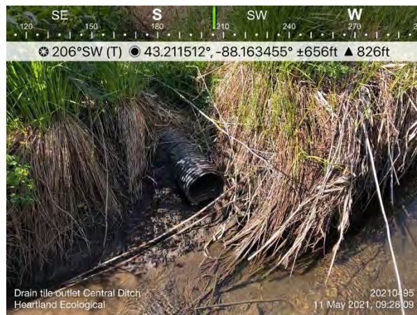
Photo #10 Photo of drain tile outlet located in the central ditch (WW-1)
