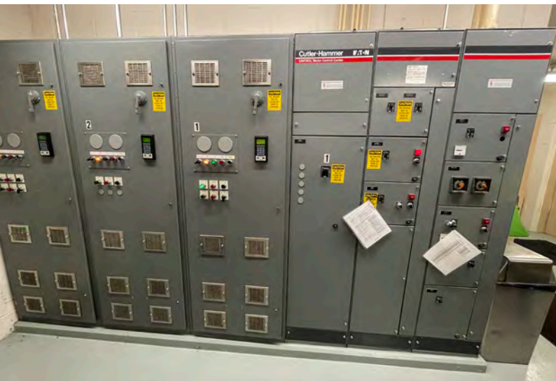
Old Farm Motor Control Center
