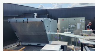
MECHANICAL, ELECTRICAL, PLUMBING, TECHNOLOGY
