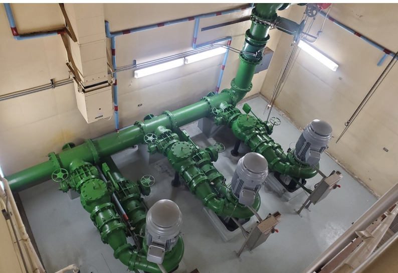
Main Street Pumps
