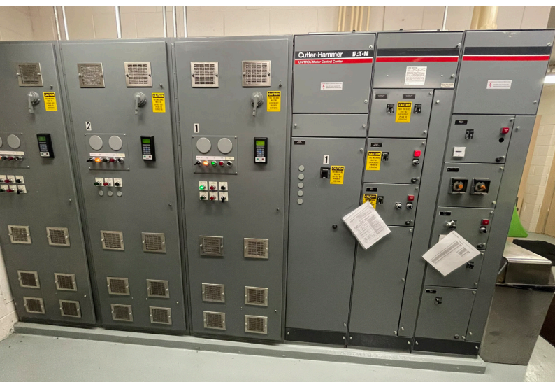
Old Farm Motor Control Center
