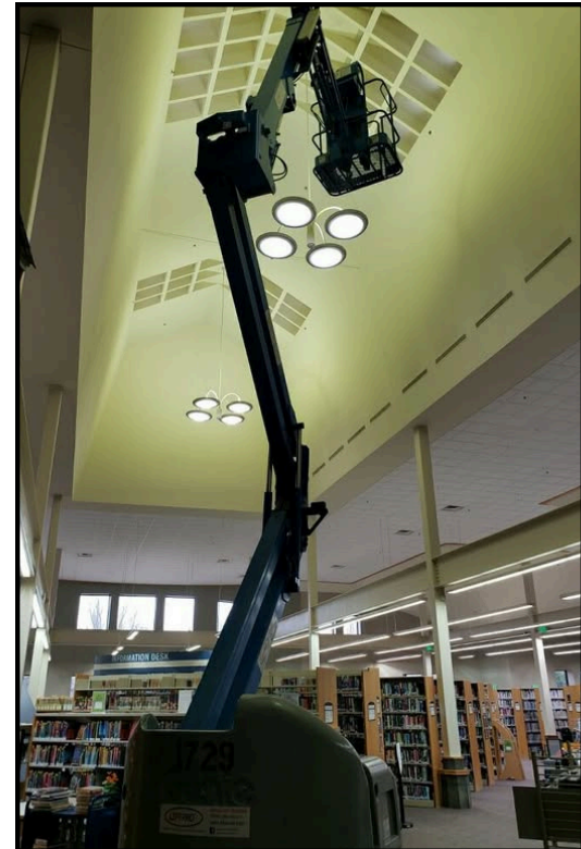
There was a lot of construction over the past few months as we completed the Door Access and Fire Panel projects
